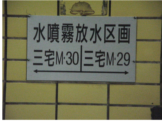
Figure D-16 Border between 2 sprinkler sections (M29 and M30)
