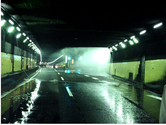
Figure D-47 Activation of sprinklers on one side
