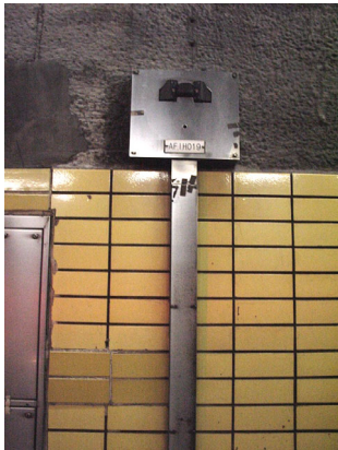
Figure D-23 Fire detector
