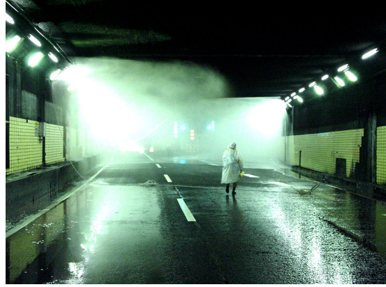
Figure D-48 Activation of sprinklers on other side
