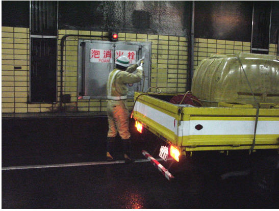
Figure D-41 Wash SOS station
