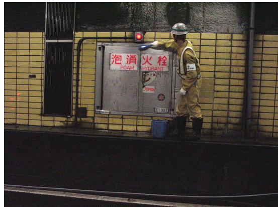
Figure D-40 Clean SOS station
