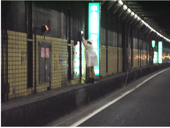
Figure D-21 Inspection of fire detector
