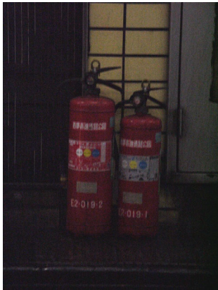
Figure D-43 Fire extinguishers
